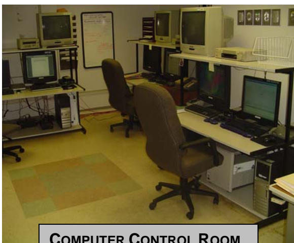
COMPUTER CONTROL ROOM
